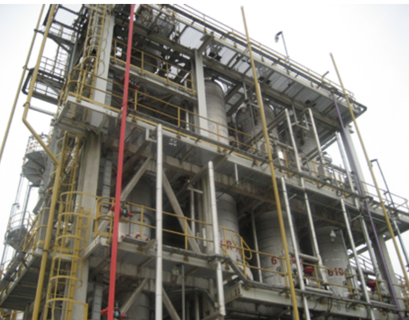
Three MP WAO reactor modules at BYC, Nanjing, China
