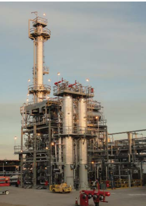
Badger BenzOUT technology at Husky Energy's refinery in Superior, Wisconsin.
