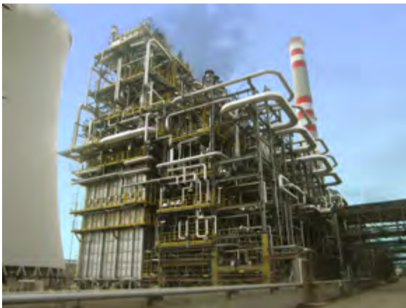
Furnace project in Europe
