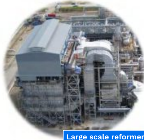
Large scale reformer
