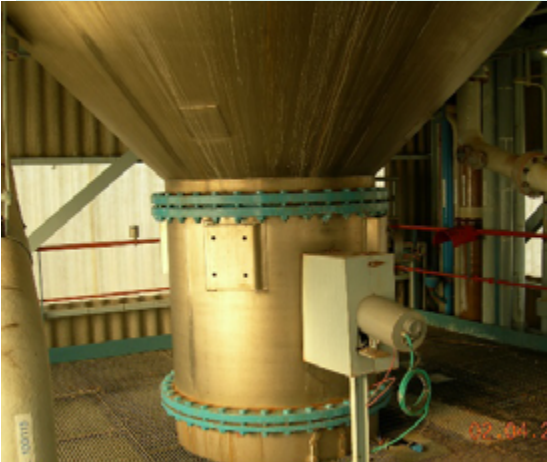
Chlorination reactor in Arkema plant (France)
